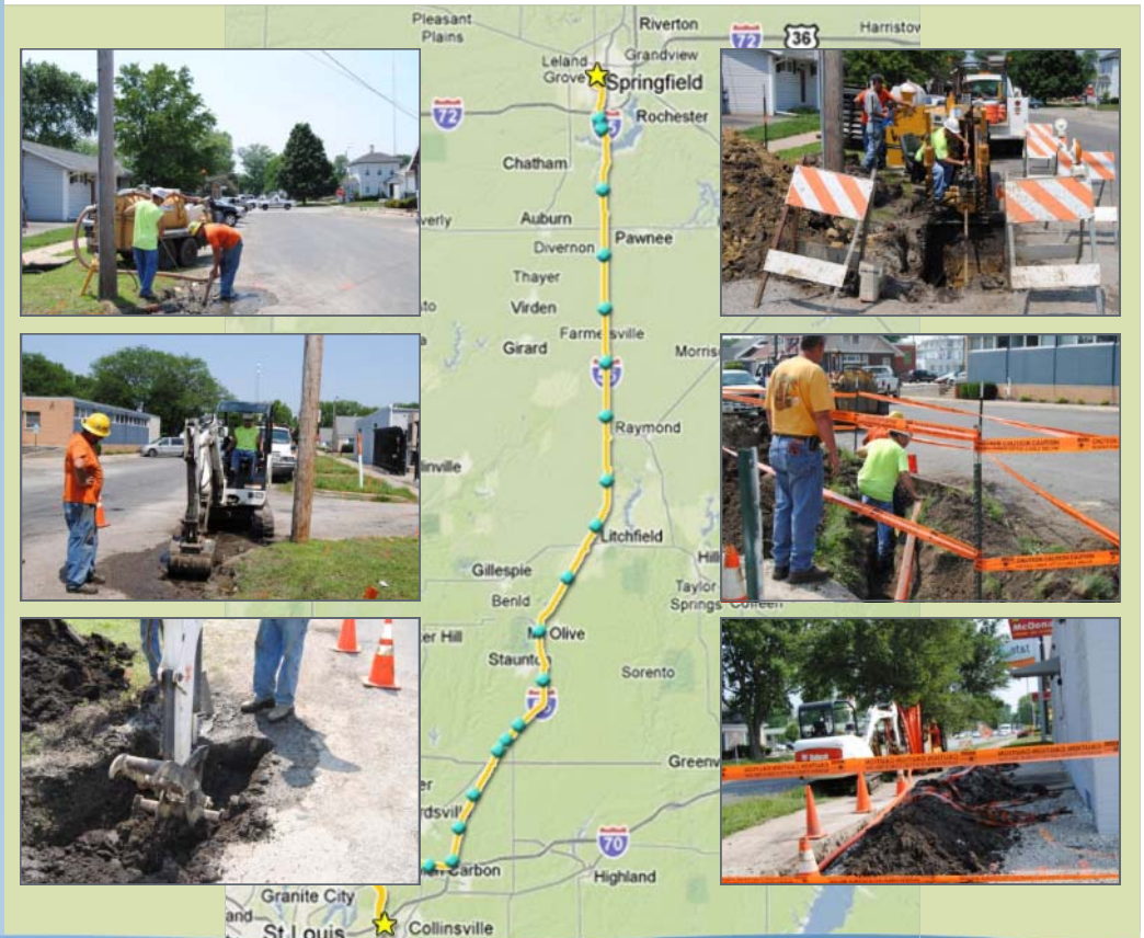
Pictures to extend leased fiber into the ICN POP site in Springfield, Illinois.
